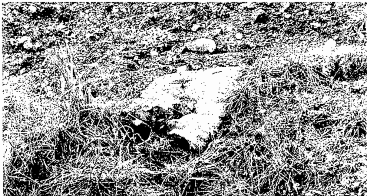
Figure 137 - Poorly protected culvert
