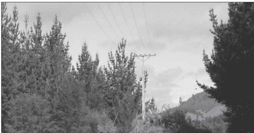
Easement agreements are essential when lines are upgraded The more power going down the line, the greater the potential liability for an outage
